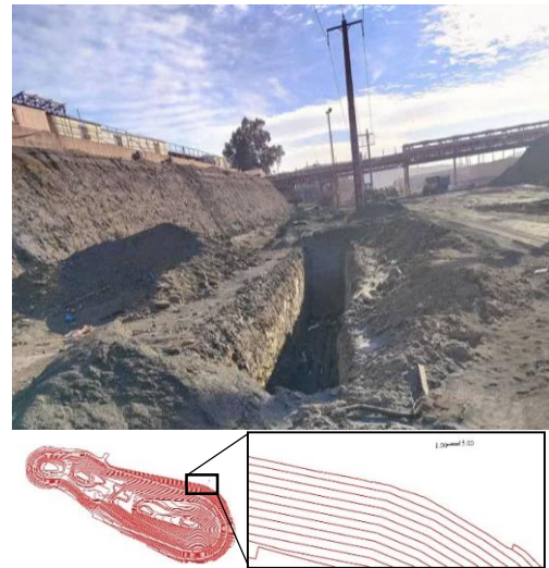
Fig. 13. Excavated trench with dimensions 15m by 1m and a depth of 3m, and its position relative to the Gol-Gohar Sirjan mine.
